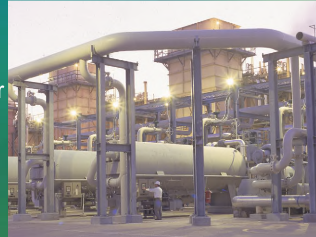
Calpine Clear Lake Cogeneration
